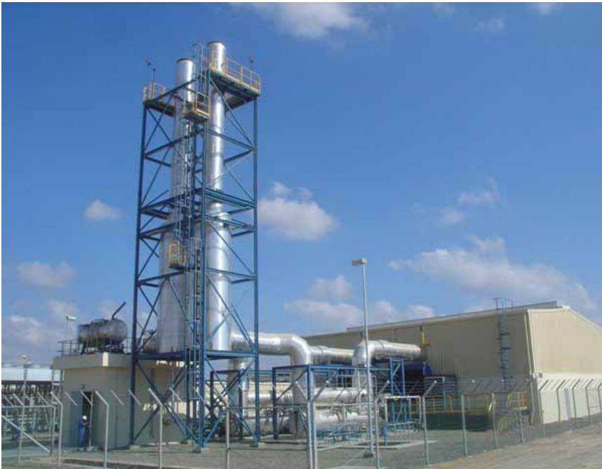
Phase 2 of the Marsa Alam power plant has been handed over by EN
